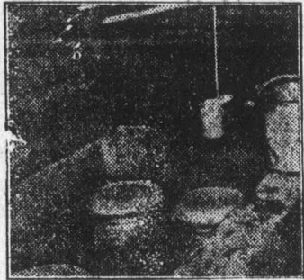
Concrete Tank for Cooling Milk.
