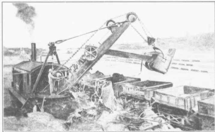
THE FREIGHT YARDS —This photograph shows part of the Pontville freight yards and the already leveled site of the G. T. P. shops.
