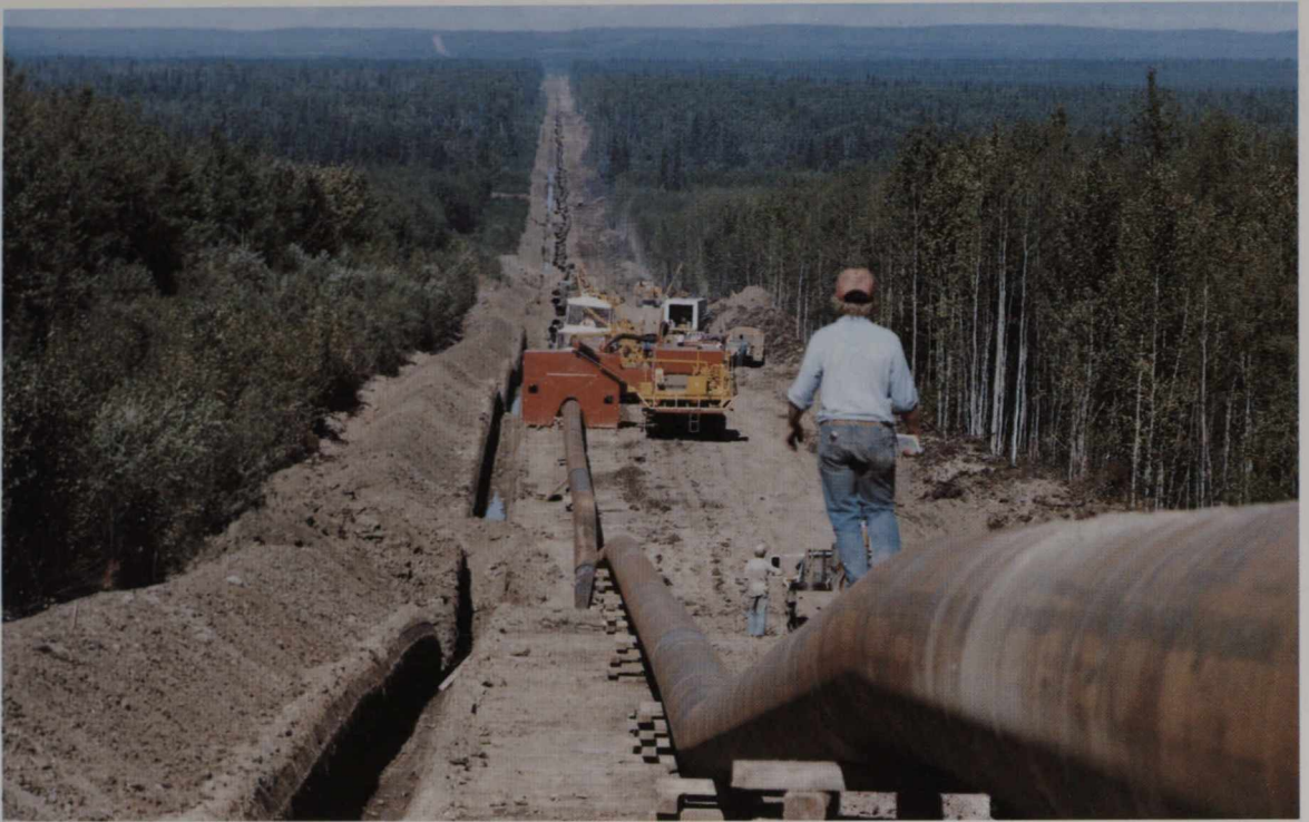
Alberta Gas Trunk Line built 80 miles of pipeline near Peace River. The red hut is a mobile welding shop.
