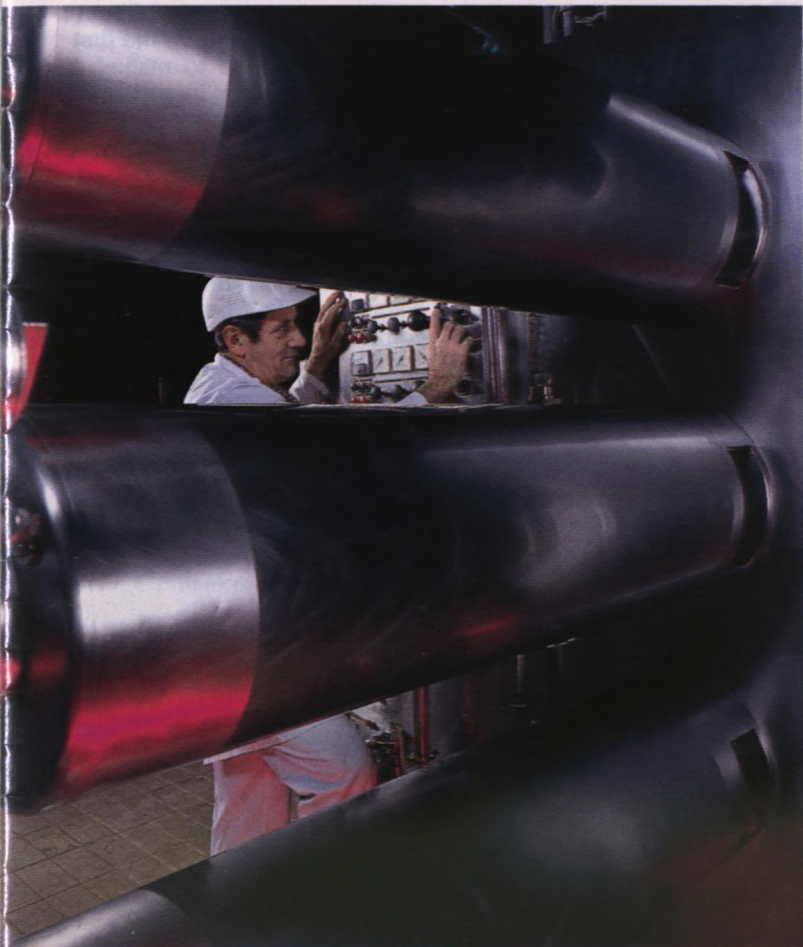
Equipment used in the waste-water purification process (waste produced by cheese production and washing water). (Coopérative agro-alimentaire Agropur)
