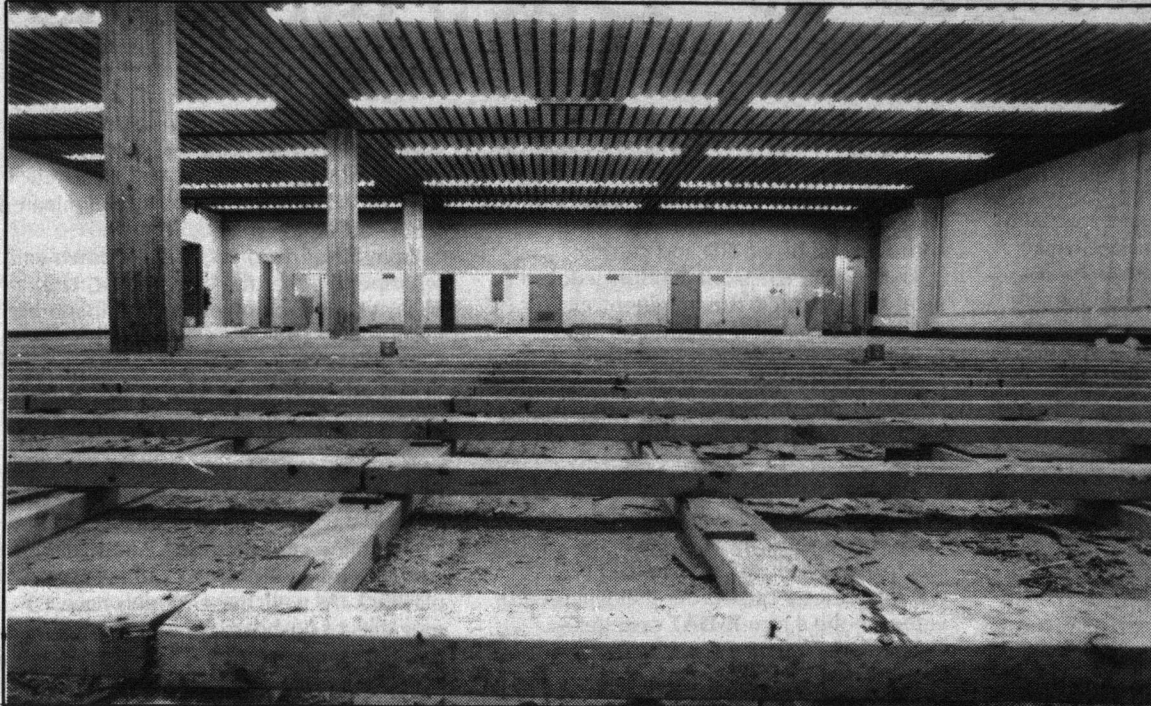
This is all that remains of SUB bowling... 2 by 4's.
