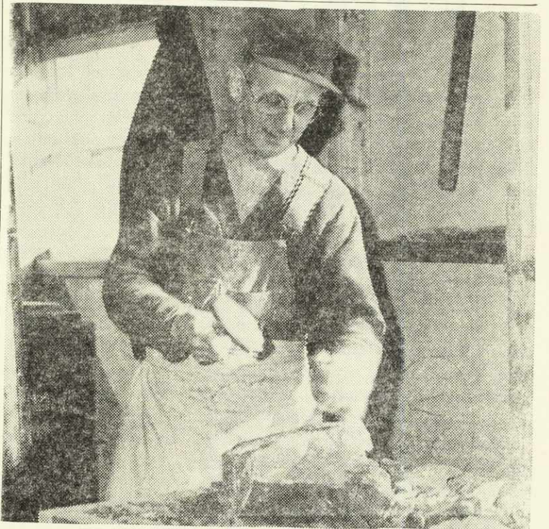
A mason is shown at work preparing stones for the new addition to Shirreff Hall. Actual construction of the new quarters will begin this spring.
