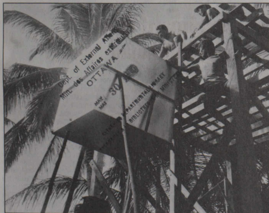
Members of SABERKAS and the community installing a water tank on the 18-foot platform
