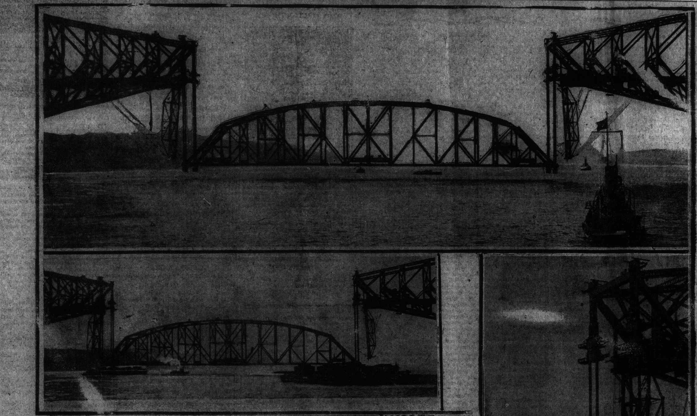
The picture immediately above shows the great span, floating on the scows, just after it was fixed into position, the mooring trusses at the side pulled back and the hoisting chains attached. The hydraulic jacks are seen on the lower level of the cantilever arms. The picture on the right shows the hydraulic jacks having lifted the span several feet towards its objective, while the central picture was taken after the span had disappeared in the waters of the St. Lawrence. The boat to the left of the chain is the government tug taking soundings in the channel, and finding that navigation will not be impeded by the mass of twisted metal lying 200 feet below the surface.
