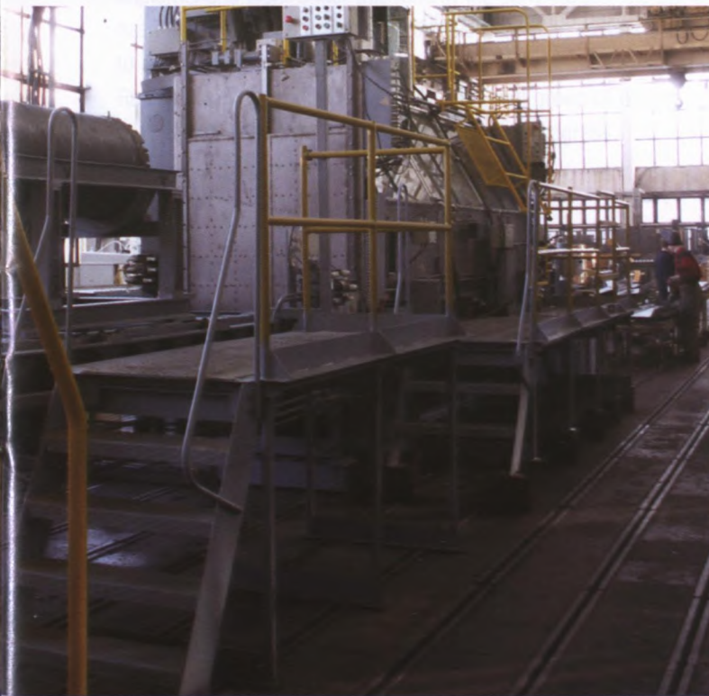
Demilitarization process line for the second main destruction building at the Shchuch'ye CWDF
