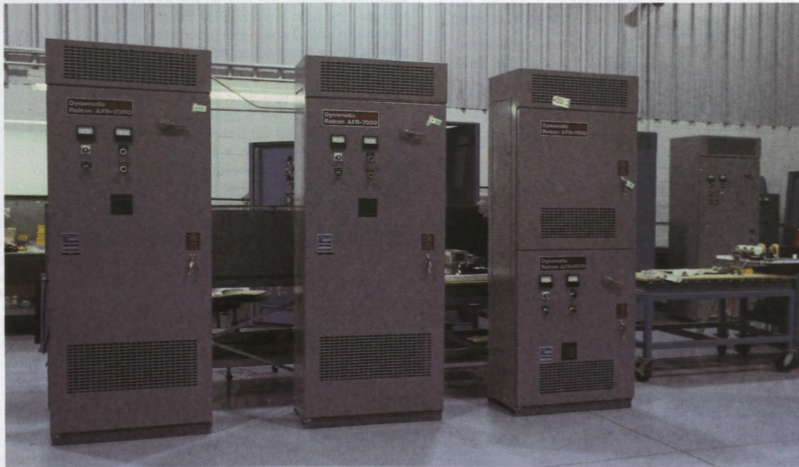
Variable torque adjustable-frequency Relcon drives are designed specifically for fan and pump applications.
