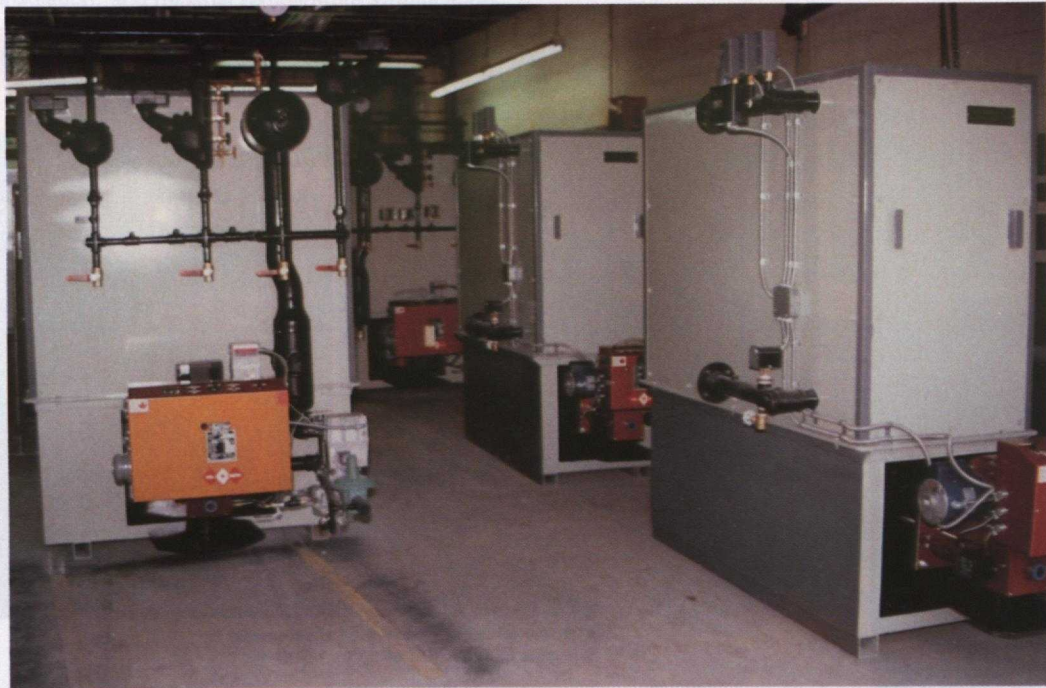
The photo shows a 6 million Btu high-pressure steam boiler on the left and two hot water boilers of 2.5 million Btu capacity each, on the right side.
