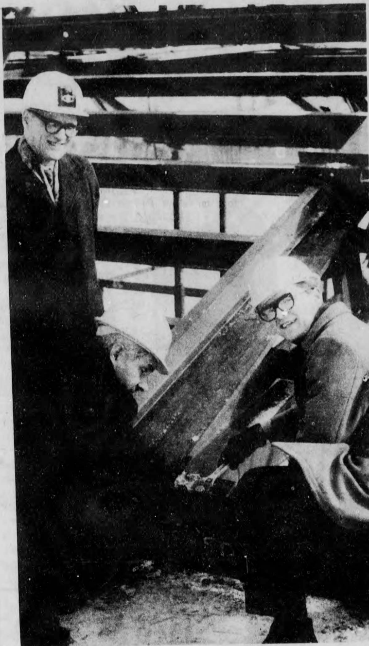
Last Tuesday a "topping off" ceremony was held at the site of the Student Union Building. The ceremony marked the placing of the last bolt in the steel superstructure of the building.
