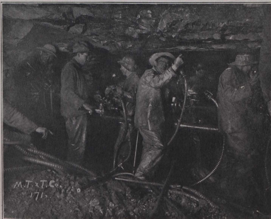
Mount Royal Tunnel—Heading. Observe Drills on Horizontal Bar and Water Attachment to Drills.
