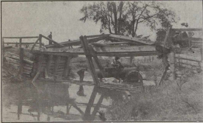
A Timber Bridge after Collapse.
