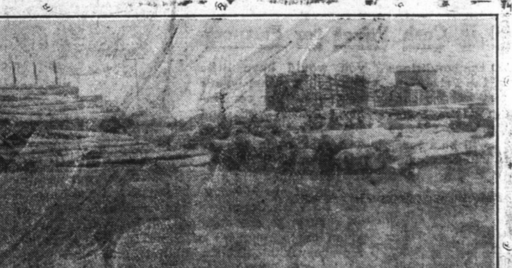
Unloading Telegraph Poles for a Stretch of 100 Miles. To be Used on New C. N. R. Line North and East of Mornville.
