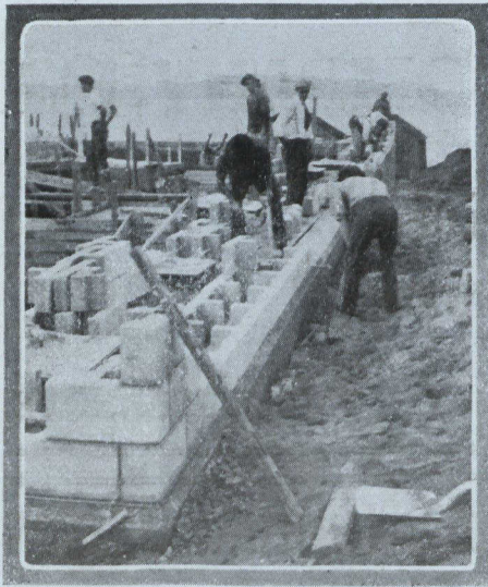
The manner of laying Hydro-stone is here shown. The workman in the right foreground is setting the pre-cast blocks in cement mortar—his helper, working inside the foundation, is placing a row of blocks in readiness for laying.
