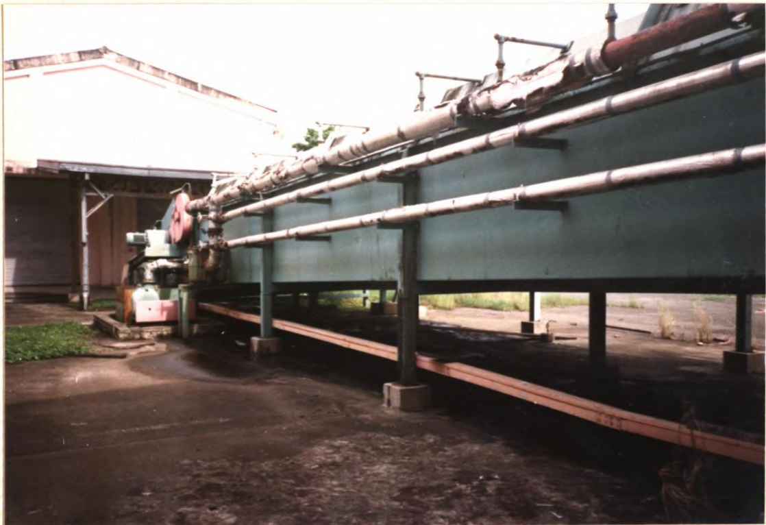
No. 14. OSB log infeed conveyor.
