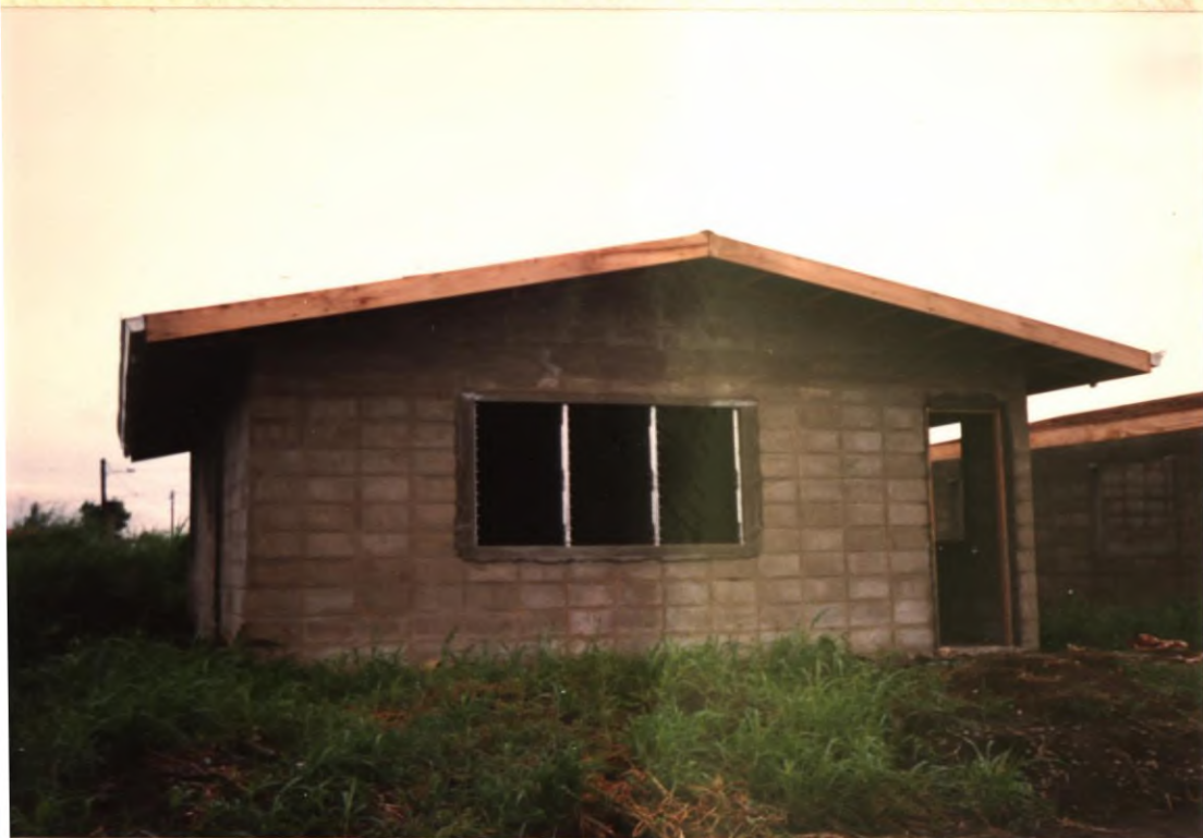
No. 67. Door and window frames installed and corrugated sheet metal roof and gutters complete.
