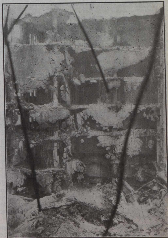
Fig. 6—Looking Directly Toward Standing 1½ Bays to the north. View taken from Standing Bays at the south end.
