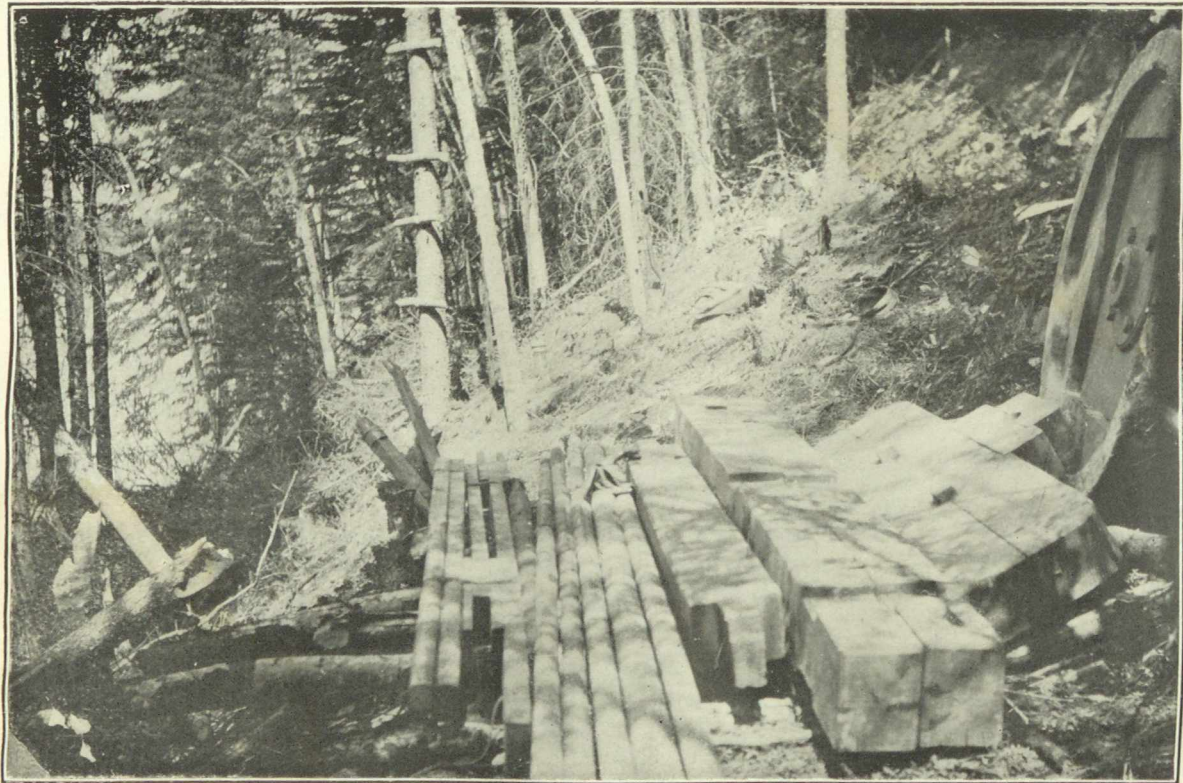
Oil boring machine in place, beyond Fort McKay. Latitude 56^{\circ}3' , longitude 111^{\circ}3' . Timber cut in locality, spruce, 18 feet by 18 inches.
