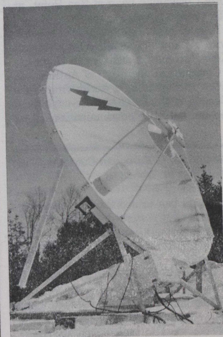
New 12-foot AniKom earth station at Northern Electric, Lucerne, Quebec.
