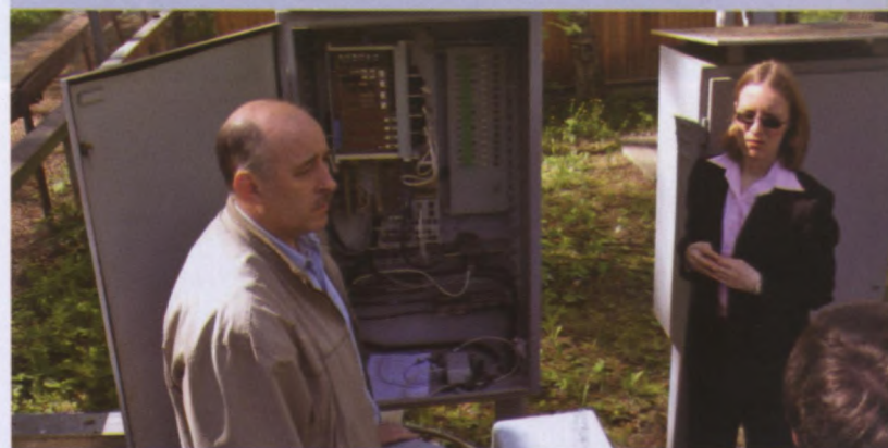
The installation of detection sensors and cameras along perimeter security fences is a key measure to help prevent the theft of dangerous nuclear materials. Photo Credit: Obninsk Interdepartmental Special Training Centre
