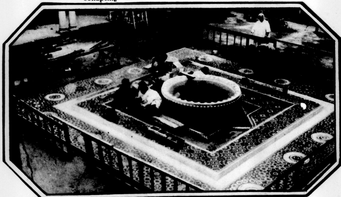
Arab workmen, imported from Africa, laying Oriental mosaics in the Mohammedan mosque being built in Paris
