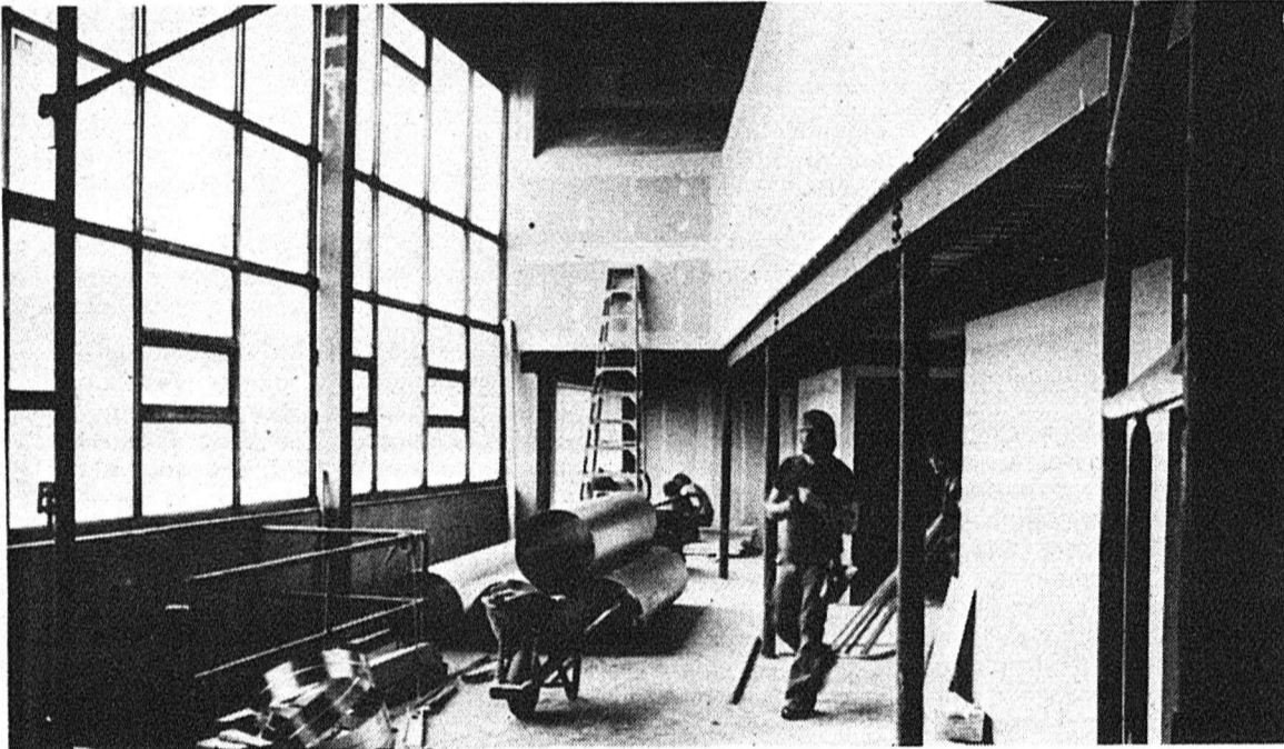
From shack to stage: The walls take shape, and, in time, the new Theatre 3 auditorium will be providing Edmontonians with unique theatre.
