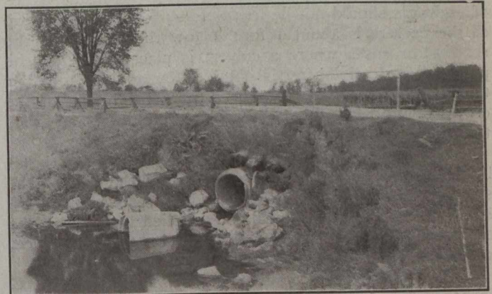
What Happens when Good Endwalls are not Used and Pipe not Properly Located.
