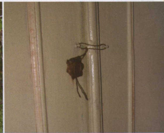
Canada is supporting physical improvements at certain vulnerable biological facilities, where dangerous pathogens are at present “secured” with string and wax seals.
