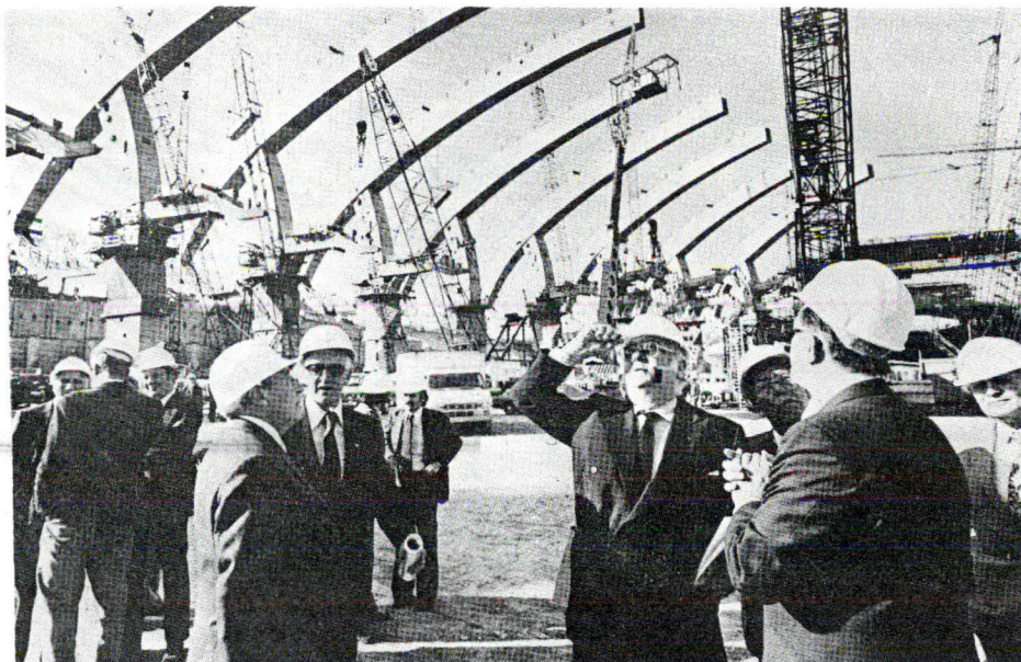
Lord Killanin, president of the International Olympic Committee, inspects construction progress on the Olympic
