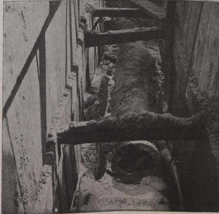
Fig. 1.—Showing Canvas Cover in place on bell end of pipe, ready for spigot end of next pipe. This view shows the efficiency of these covers. Note the water in the trench, kept out of pipe by the covers over the joints in background, which are concealed under 3 inches of concrete.
