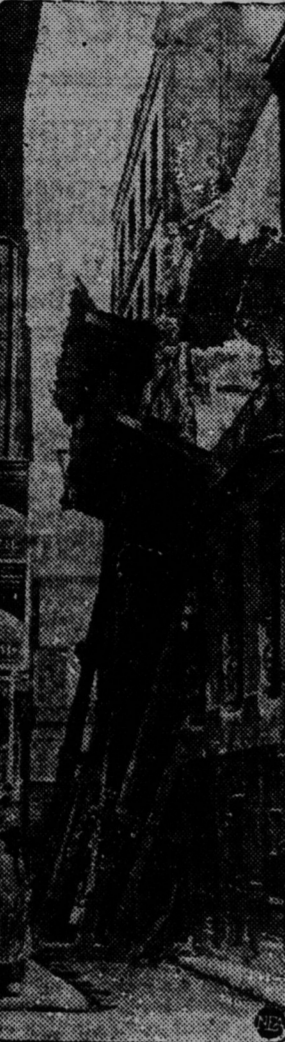
Workers have just begun tearing down this Paris tenement, damaged by German bombers. "Big Bertha" shelled the French capital during the World War.
