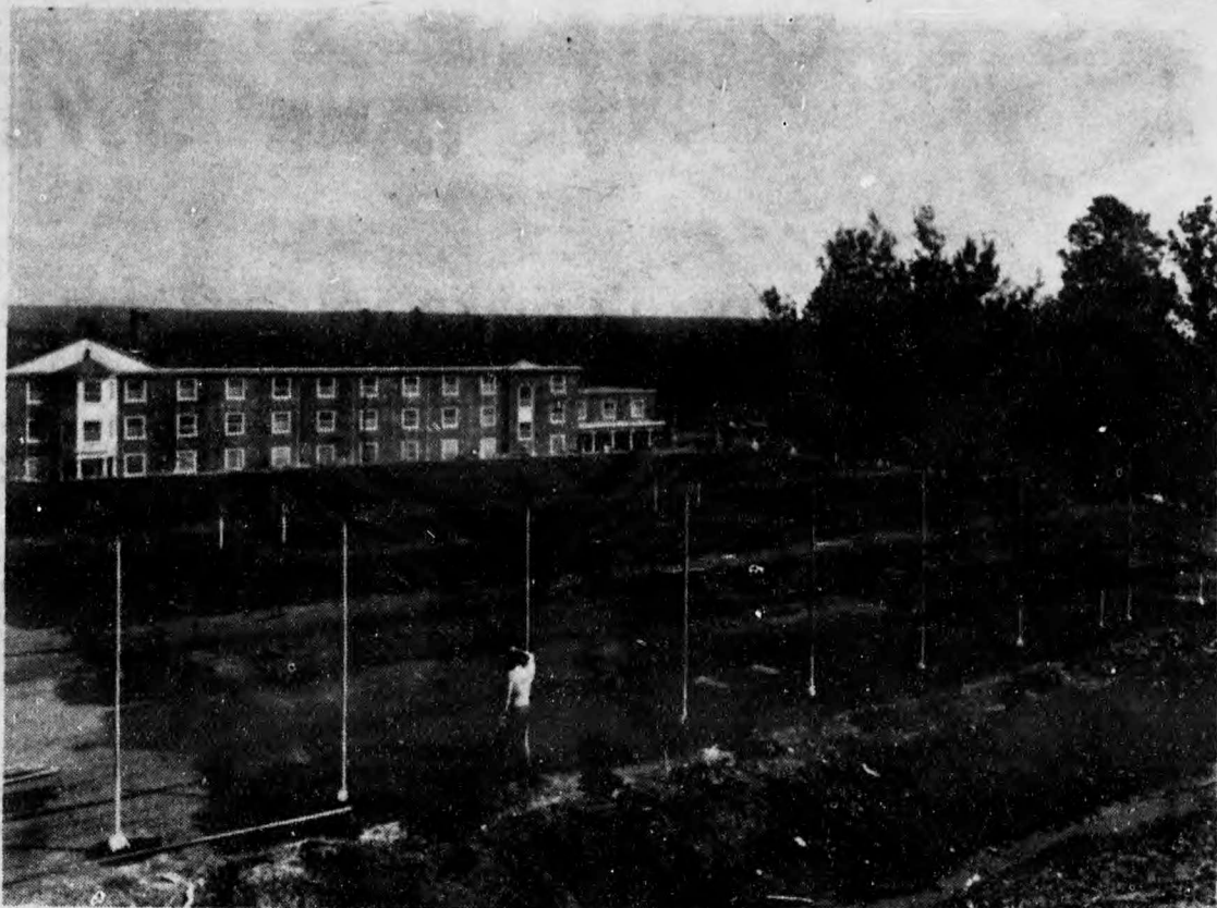
The newly constructed tennis courts beside Lady Dunn Hall should be ready for their first matches soon. The courts were to have been ready for summer school, but work has been held up until now.
