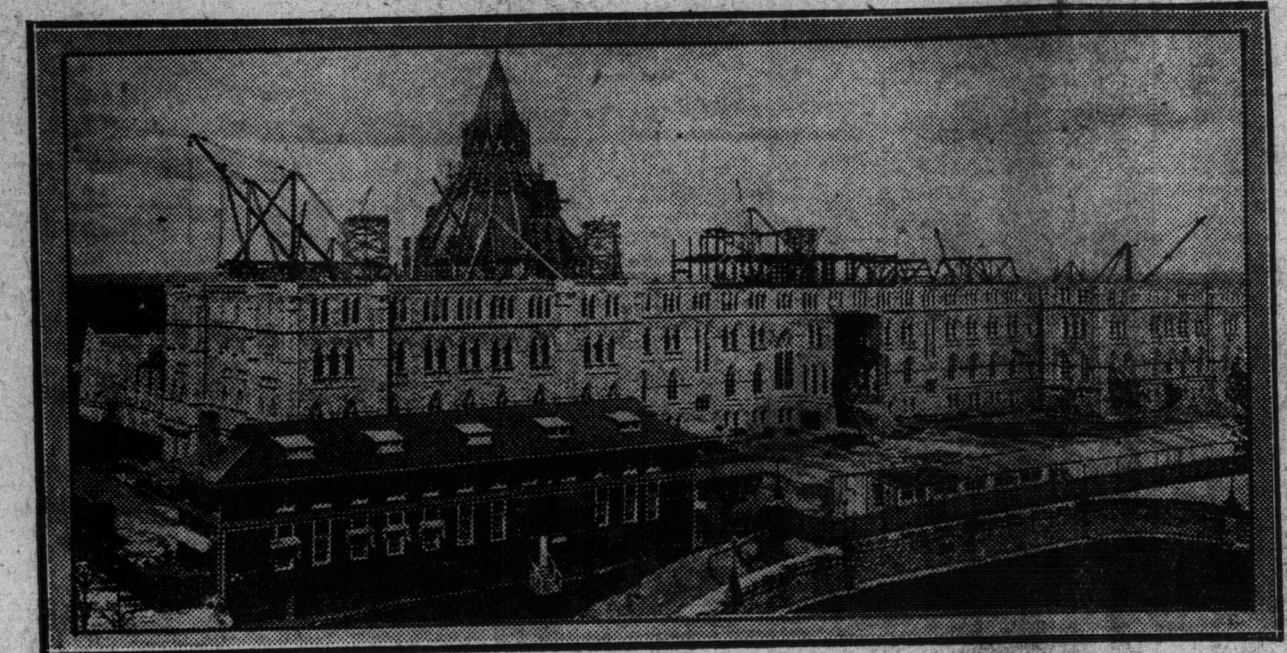
Photograph showing progress made on the reconstruction of the parliament buildings at Ottawa. Work was started one year ago, and as of now work done during the winter this represents eight months' building.
