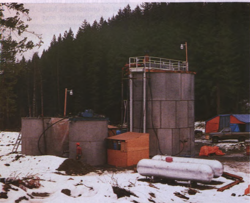
The largest biological leaching reactor in the world. The tank measures 6.5 m in diameter and 7.2 m in height. This reactor is located near Goldbridge in British Columbia.
