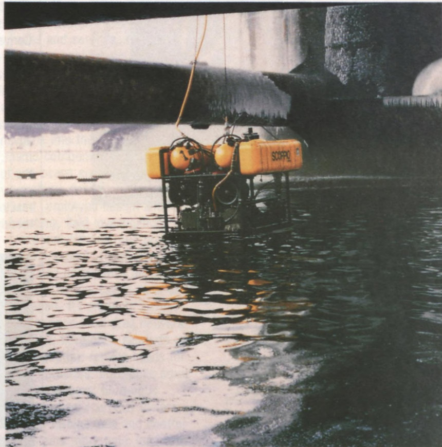
Dominion Diving specializes in drill rig support, marine construction and in-water repairs.
