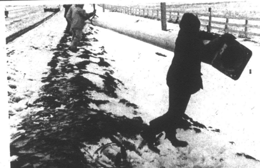
Three new aluminum light standard poles came crashing down onto Highway 10 during a wind storm. As a safety precaution the remaining 37 poles were removed.
