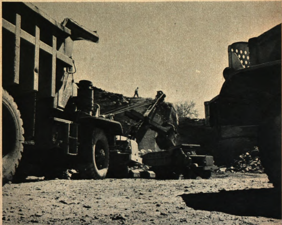
Excavating blasted rock in the Côte Ste. Catherine cut, site of the Seaway lock and twenty-seven-foot channel opposite Montreal
