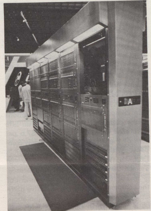
Northern Telecom Limited's DMS-100 (digital multiplex system) switching machine featured in the corporation's exhibit at Telecom 83. This is the first appearance of a working model of this large central office machine at a trade exposition. It has a capacity of up to 100 000 lines and will be used to demonstrate the capabilities of the machine as it relates to various systems in Integrated Business Networks, integrated voice and data terminals, Autovon military network, Maintenance and Administration Positions (MAP) and Traffic Operator Position Systems (TOPS).
