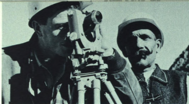
A Canadian engineer, with his Pakistani tribesman assistant, at the site of the Hydro Electric Project at Warsak, Pakistan.
