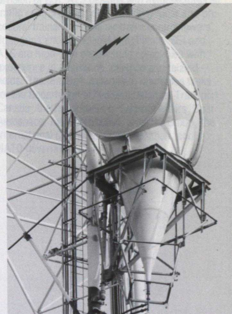
Microwave communications antenna system
