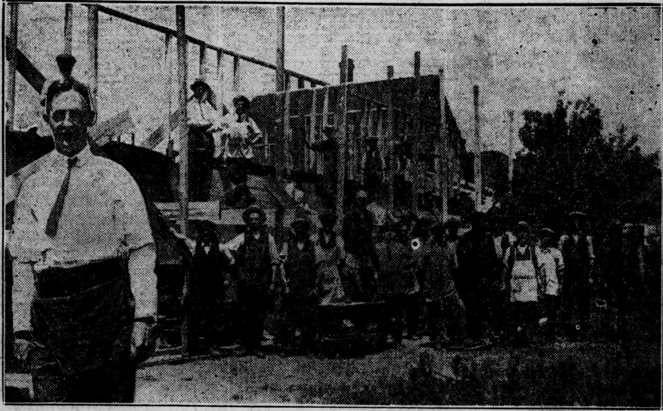
By The Free Press Photographer. The members of St. David's Anglican Church are building their own parish hall. The carpentry work is being done by the men of the congregation, and on the holiday there was no end of helpers.
