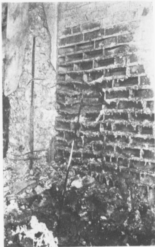
Fig. 19. Melted brickwork in concrete warehouse.
