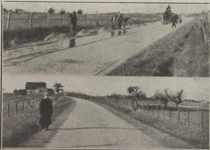
Fig. 2.—Edward VII. Road, Parish of Napierville. (Upper) Laying Gravel on Fluxphalte. (Lower) Finished Road.
