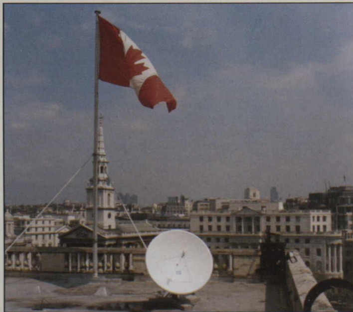
Norsat receiving dish recently installed on the roof of Canada House in London.
