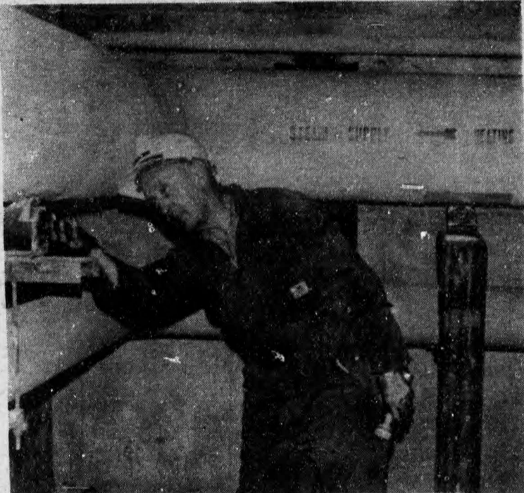
A UNB employee checks the pipes in one of the university's many tunnels. PHOTO BY DEFRIETAS
