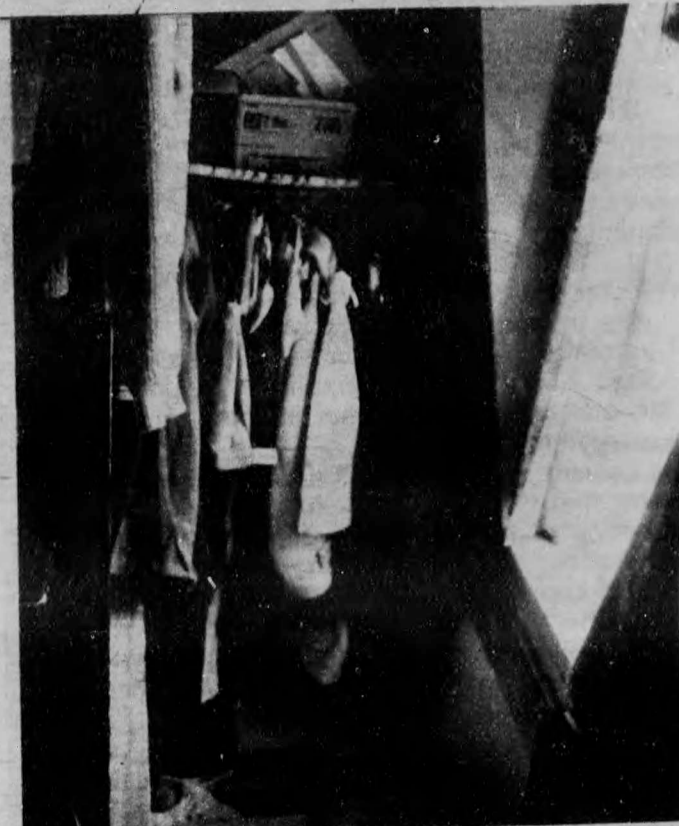
The landlord of this apartment has blocked the fire exit to form a closet. - Photo by Wallace.
