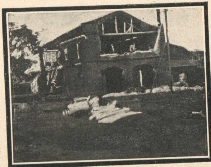
A Building wrecked by the Earthquake.
