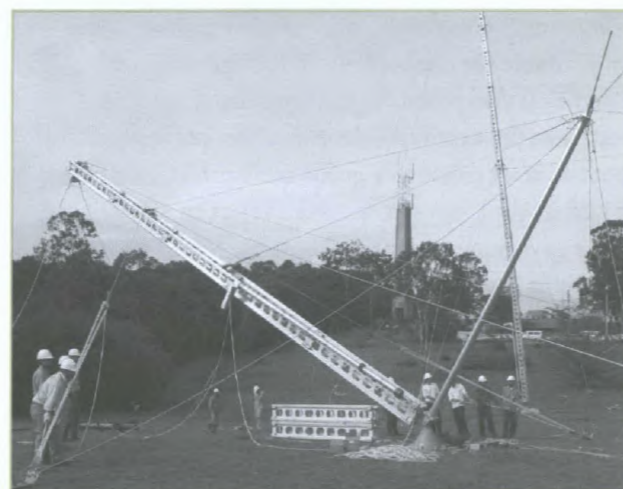
SBB International's emergency electrical towers
