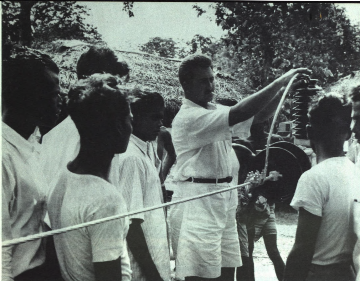
A Canadian transmission engineer demonstrates mechanised methods of transmission line construction in the Gal Oya Valley, Ceylon.
