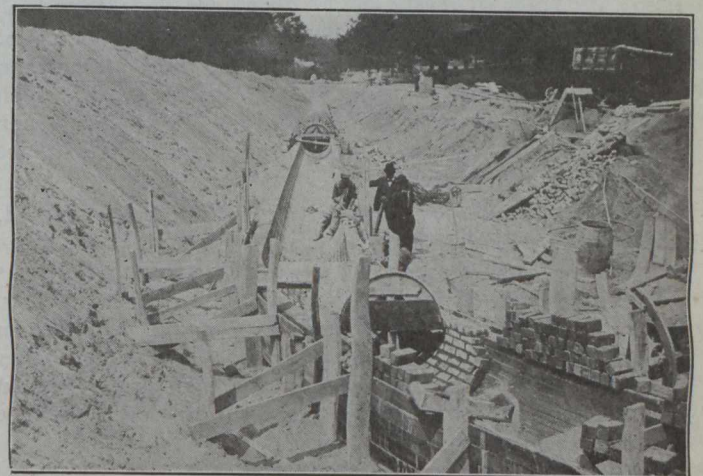
Material was Dumped Over Banks of the Fill Instead of Being Raised by a Donkey Engine
