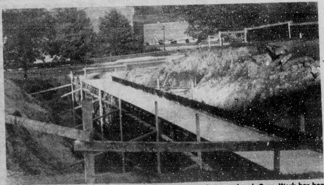
To cure the problem of leaky steam pipes leading to the Lady Beaverbrook Gym, work has been going on over the last few weeks to install a new tunnel. The work should be finished by the end of October, but while it is in progress it will be necessary to close the road for a while in the next couple of weeks.
