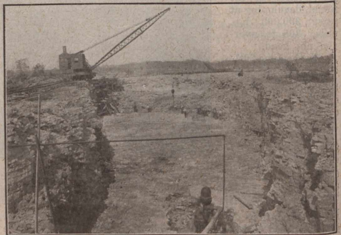
CRANE MOVING ROCK IN SKIPS FROM CANAL SECTION AT ENTRANCE TO FOREBAY
